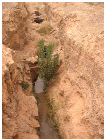
27m length was completely damaged by floods.
