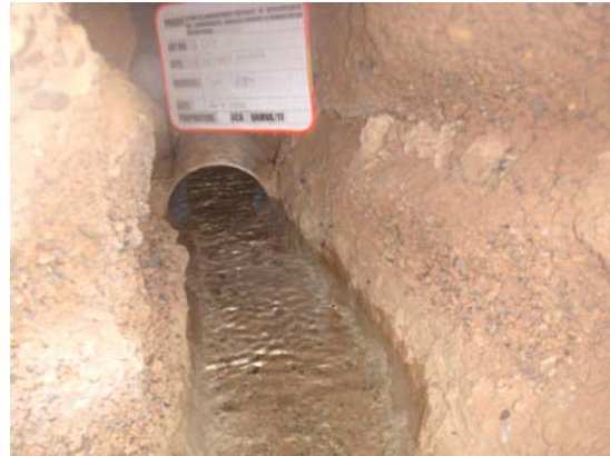
Most upstream of PVC pipe Pipe diameter has certain surplus flow capacity for increase of discharge in future.
