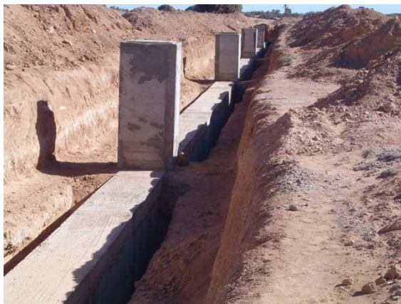
Gallery and vertical shafts of interval 30 m ( Middle portion of total rehabilitation length of 300m
