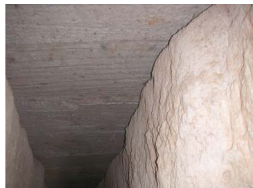
Replacement of gallery cover by concrete slab. (see from inside of the gallery)
