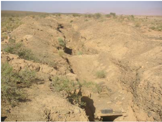
Before rehabilitation works. Masonry wall of gallery was damaged by flood.
