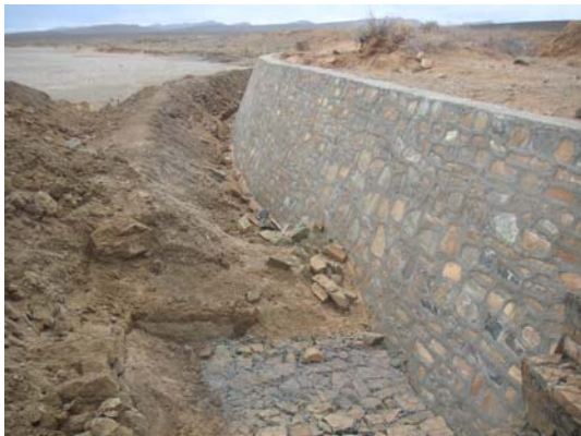
Flood protection dike is effective to prevent the gallery from collapse or erosion in the case a gallery is situated closely to the river.
