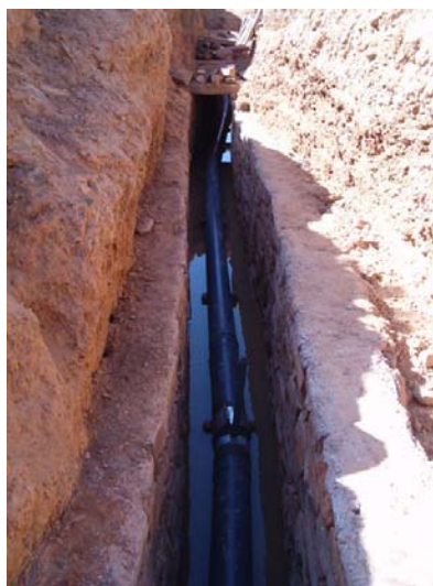
After rehabilitation works by masonry wall. PVC pipe was installed to prevent leakage.
