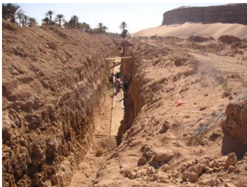
Excavation to the gallery foundation Concrete placing was commenced after open excavation works.
