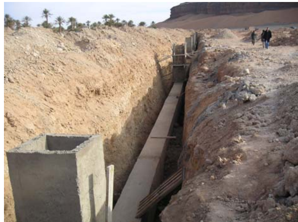
Concrete placing (gallery and vertical shafts) Gallery and vertical shafts of its interval of 30m
