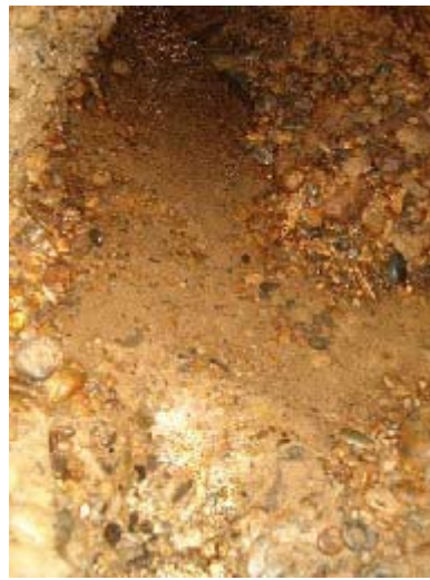
When digging to perpendicular direction In the gravel layer, water spring much.
