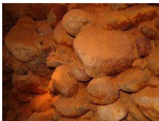
Gravel and boulder layer condition forming the portion seepage groundwater.
