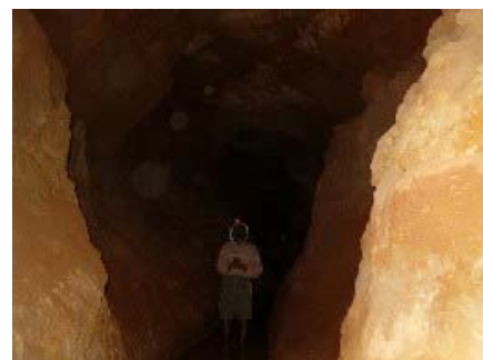
Condition of the midstream. Because the lithology around khettara consists of not bedrock but loose soil, its section area becomes much wider due to collapse of side and top wall.
