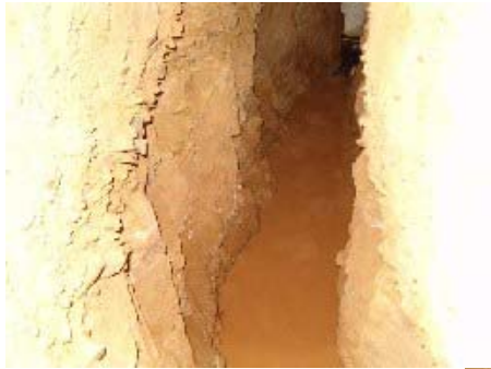
Condition of the upstream. The bottom and lower side wall is bedrock. Upper sidewall is talus or weathered rock creek formation.
