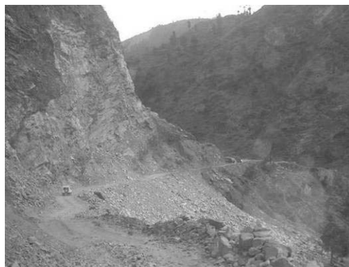
Large scale slope failure on provincial highway in NWFP, Shinkiarai - Nawab Abad Road in Mansehra District
