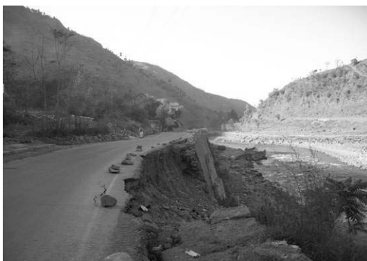
Collapsed stone masonry walls
