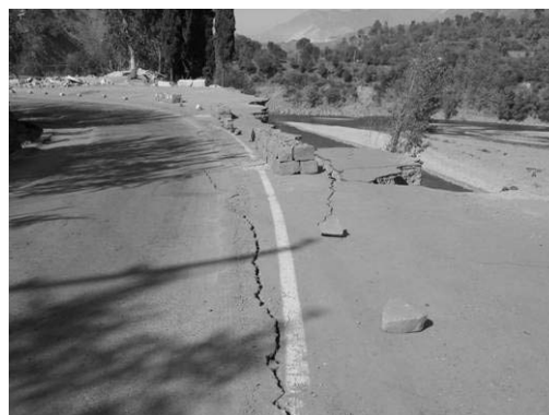
Failure of one-lane width on valley side
