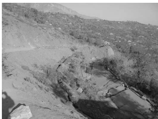
N35: Collapsed roadway by landslide
