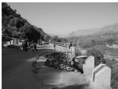
Damaged bridge approach
