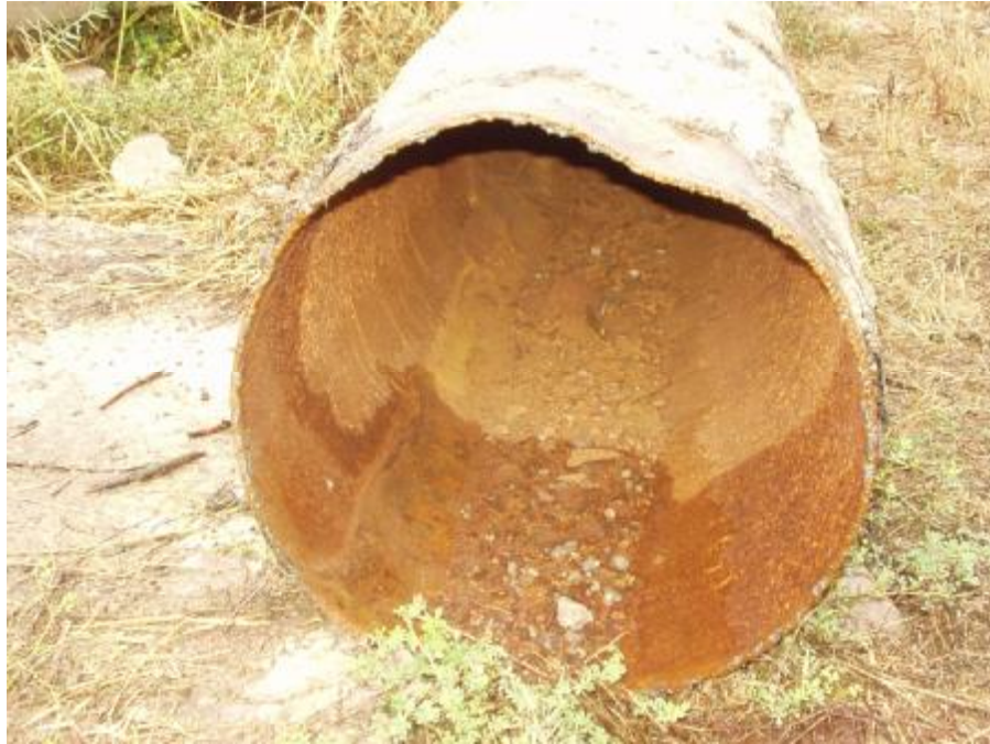
Photo S 3.1.4.1 Inner Surface of Removed Pipe
