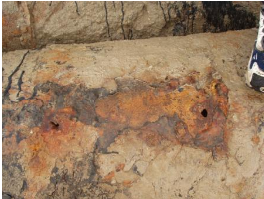
Photo S 3.1.4.2 Outer Surface of Removed Pipe
