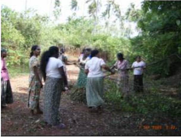
Clearance of the place by members of the society before foundation laying
