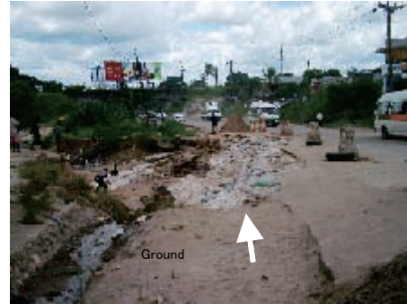
Spot of scour due to defective drainage Restoration of shoulder scoured by heavy rainfall, end of May, 2005 (water pipes, electric cables, etc. also broken)
