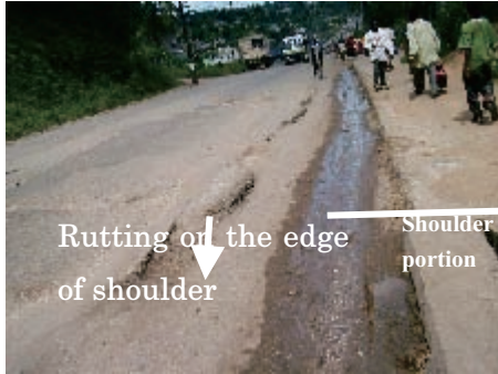
Actual state of drainage on site (Surface water flows on shoulder and has damaged the pavement.)
