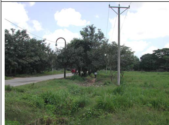
Electrical Pole in the Site
