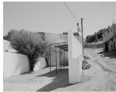
Prov. Khenifra Sidi Yahya Ou Saad Construction of fence and entrance covered way
