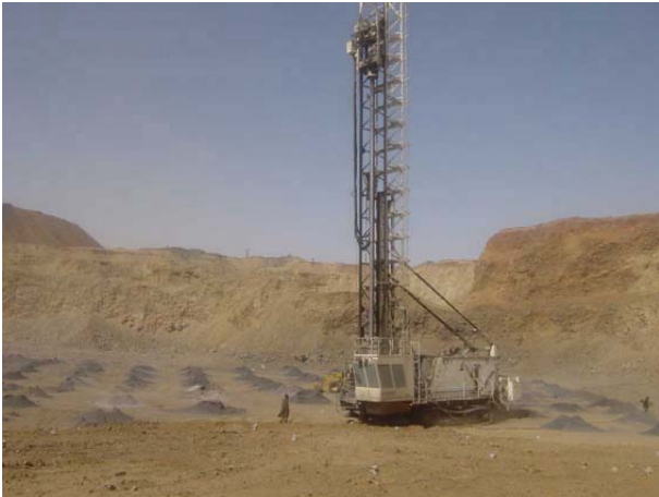
3. Drilling Work in El Rhein Mine (Depth: 18m) 3,000 tons of ore are broken by blasting of 1 tons of ANFO in each hole.
