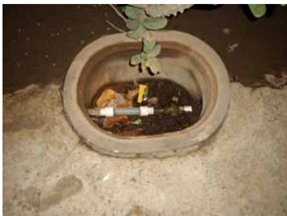
Photo 11 Direct Illegal Connection
