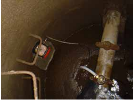
Photo-5 Pressure Recorder Installation on Pipe
