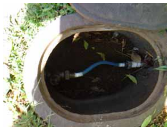
Photo 12 Direct Illegal Connection with hoses
