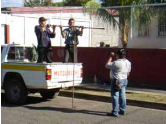
Photo-1 Boundary Valve Check for Isolation
