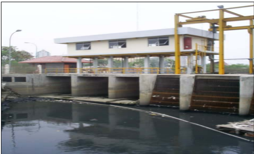
Figur 7. Bendungan Jago Sluice gate at Serdang
