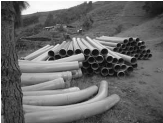
Construction with material donated to CREA by the Grass-roots Granting-Aid Program by the Embassy of Japan
