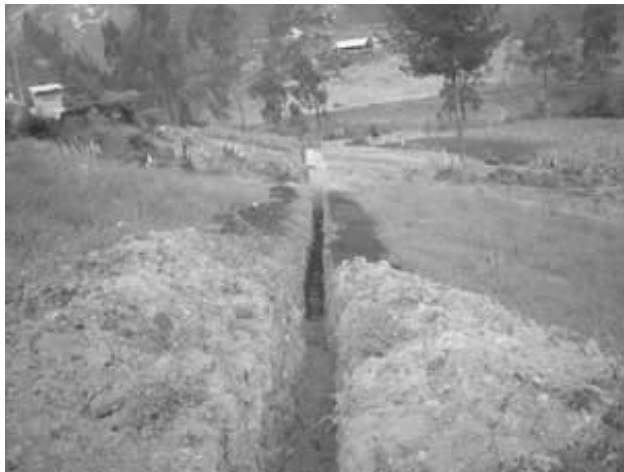
Joint project for the excavation of the water channel among residents and CREA through the Grass-roots Granting-Aid Program
