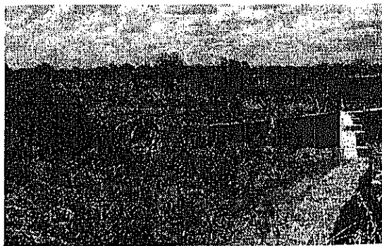
Unfinished construction (Nangaramo, Masasi)
