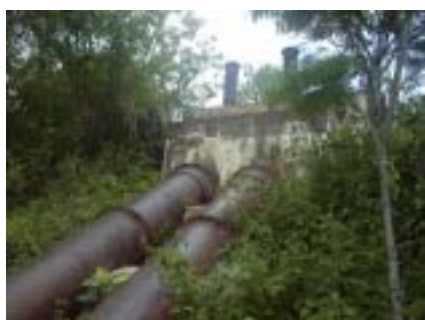
Penstock of Open Type
