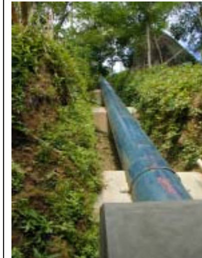
Penstock of Open Type
