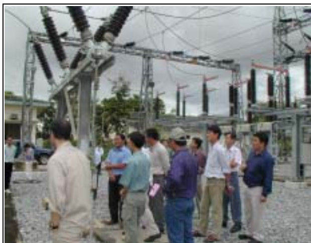
Photo-13 (July 21, 2004) Visit of Thalath Substation
