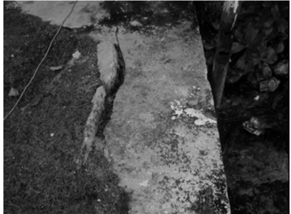
Damages of concrete at west side pier
