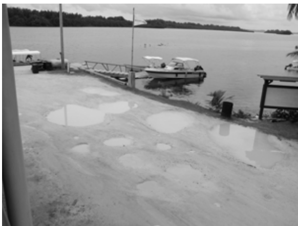
Puddles at apron after raining
