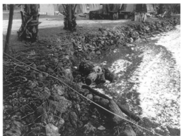
Gabions are broken and filling stones are scattered
