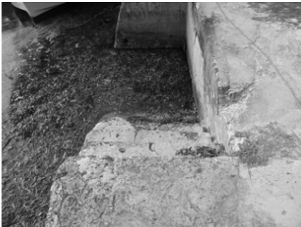
Damages of concrete at west side steps of pier
