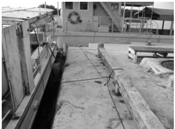
Damage and deformation of Mooring beam
