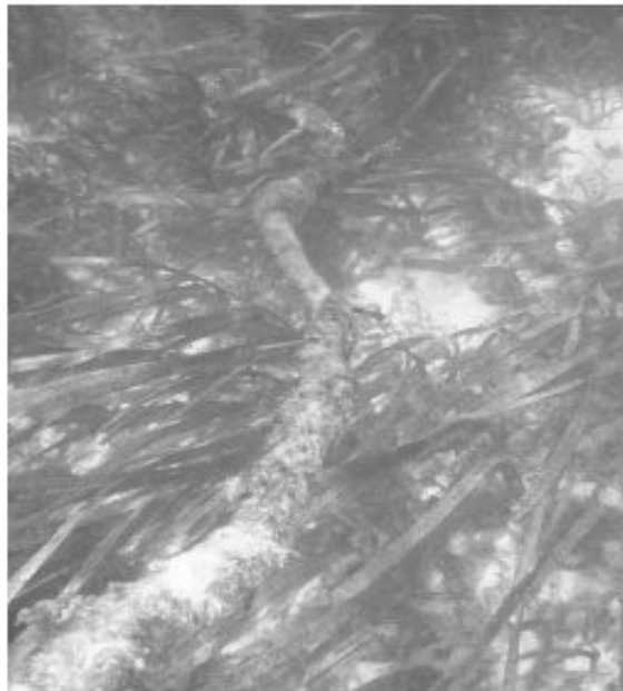
Submarine Cable pulled out of seabed, Main Channel.
