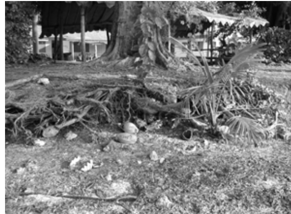
Photo2.1.3(2)-22 Eroded Tree at 20m from Pier
