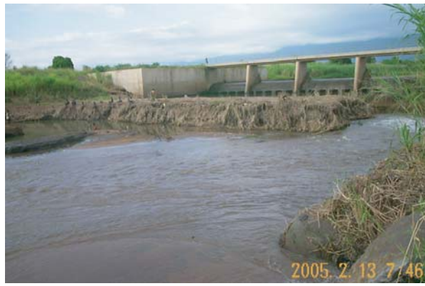
① Downstream of the Headworks (2005.2)
