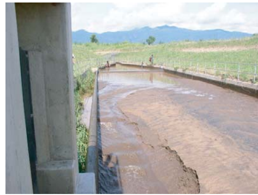
③ Sedimentation in the Settling Basin (2005.2)
