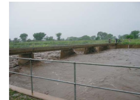
② Headworks in the flood on Feb. 28, 2005 (2005.2)
