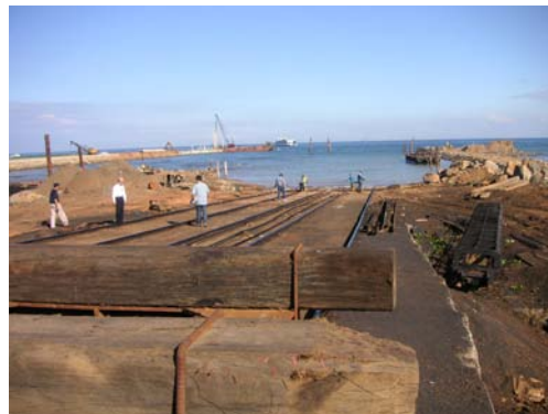
Slipway of Newly Built Seafront Shipyard
