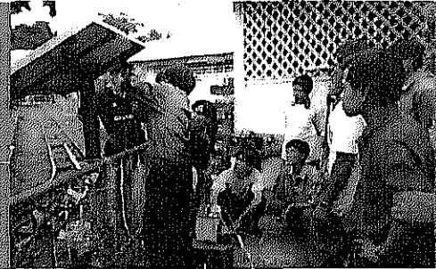
Installation of solar panels in mountainous regions where electric transmissions are difficult (Thailand)
