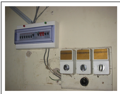
Switches on the walls are not labelled for easy identification. Also, there is only one main switch controlling all lights in an office.
