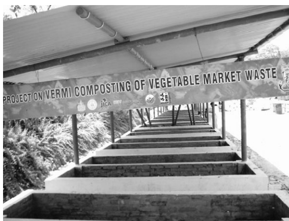
Photo 6 Cemented Vermi Tanks
