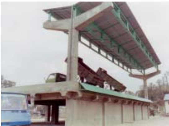
A-3: Practice of Operation of Teku T/S (April, 2005)
