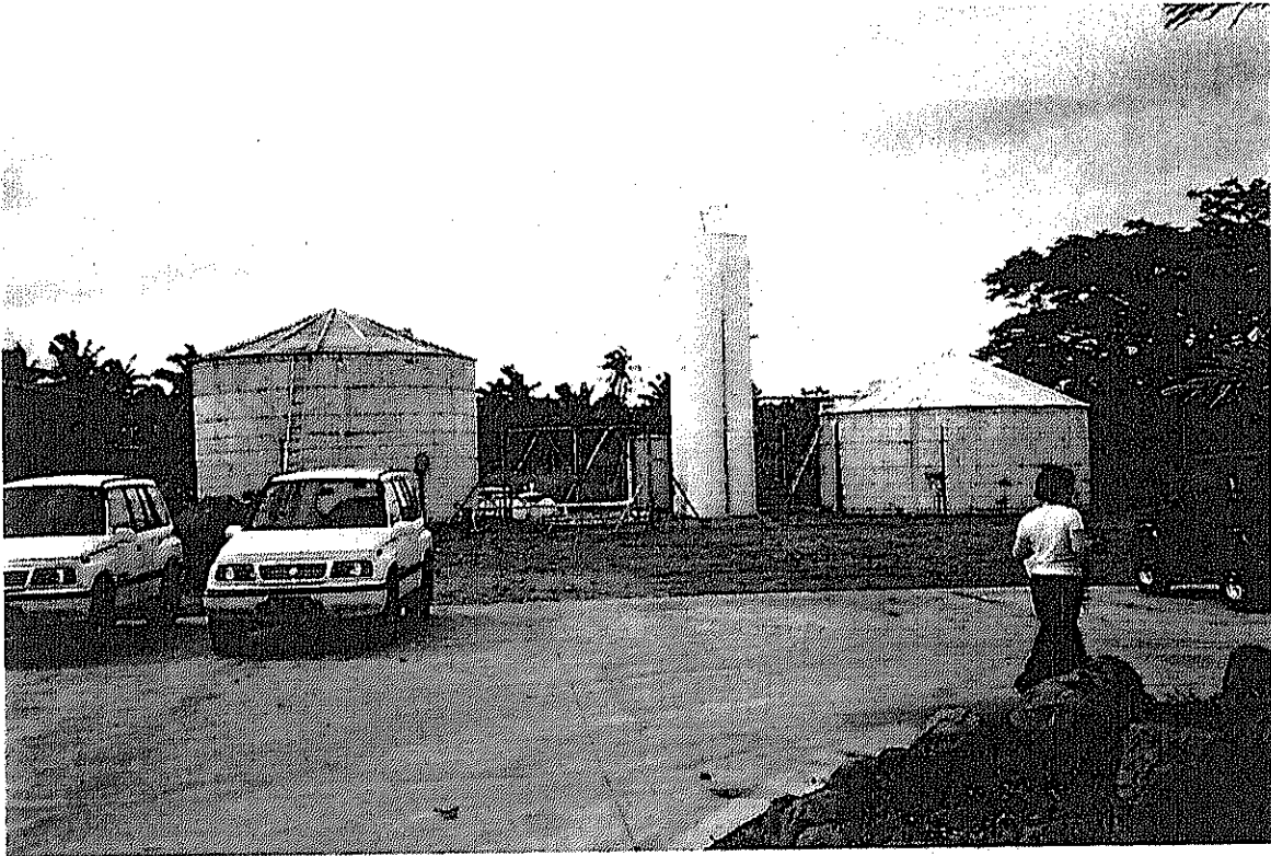
YAZAKI WASTEWATER TREATMENT PLANT - ZERO DISCHARGE (EFFLUENT RE-USED FOR TOILET FLUSH)
