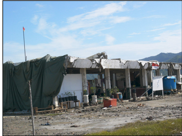
Heavily damaged SD 47
