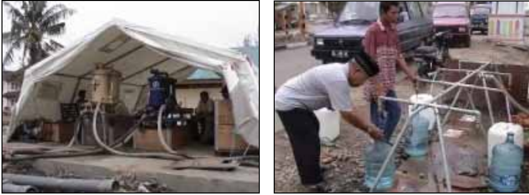
Figure 2.3 Mobile Water Treatment Equipment and Temporary Public Tap
