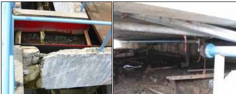
Figure 2.1 Damages in Lambro Water Treatment Plant and Primary Pipe at River-Crossing
