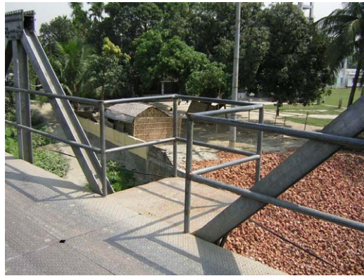
Photograph 2.2.2-1 Safety Recess provided by the Bangladesh (the Project Phase 1, Bridge Length = 115m)
