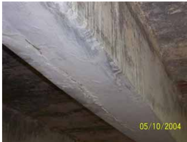
Crack in Existing Pump House
