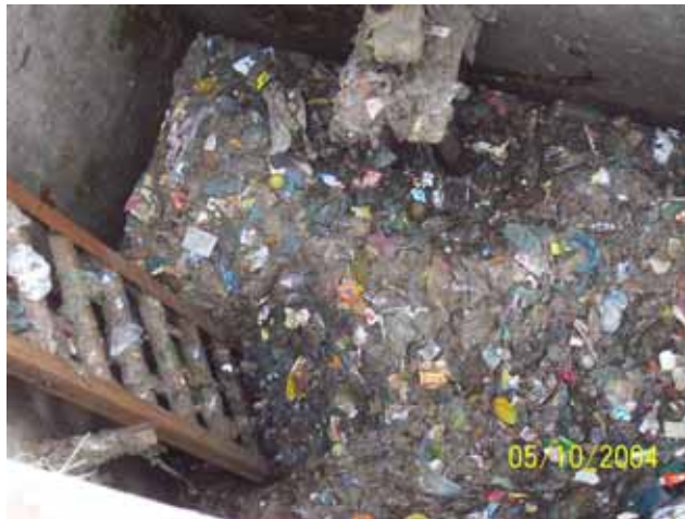
Garbage at Inlet Chamber – Gaughat SPS
