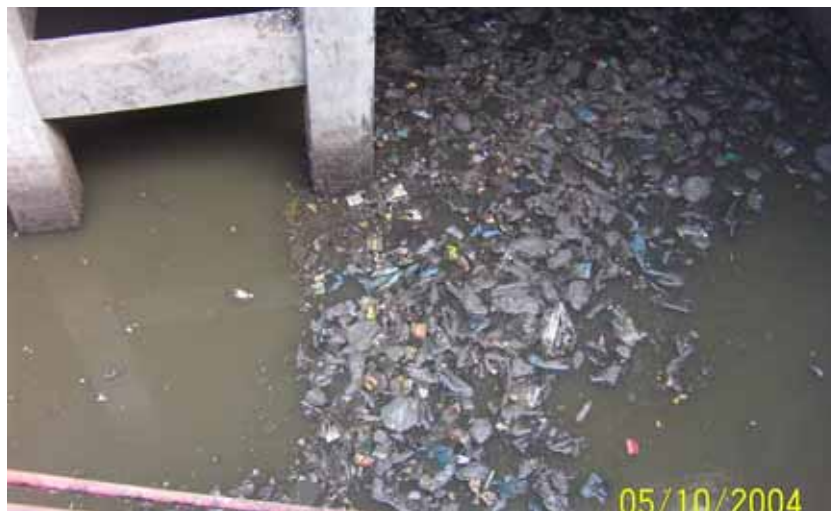
Wet Sump – Gaughat SPS
