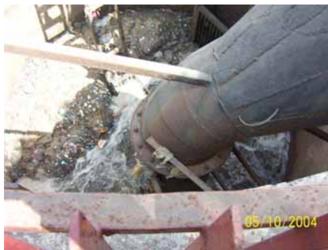
Inlet Chamber at Gaughat SPS
