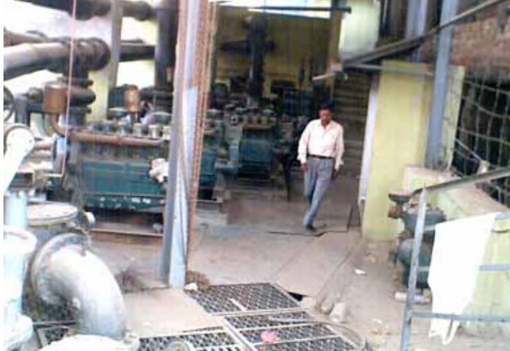
Existing Submersible Sewage Pumps at Morigate
