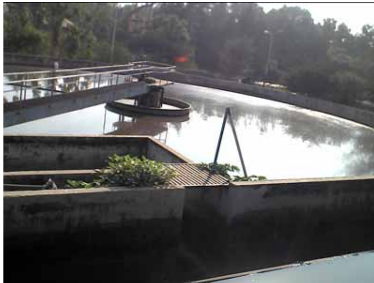
Primary Settling Tank
