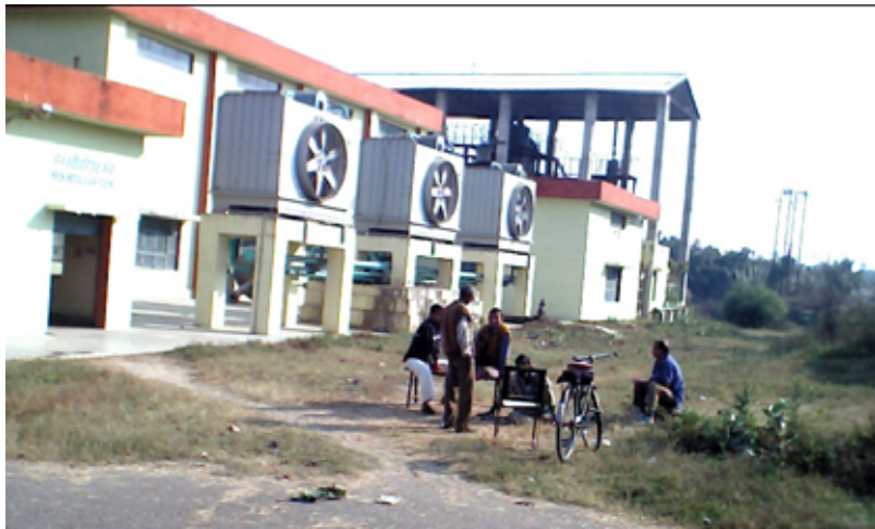
Dual Fuel Engine Room
