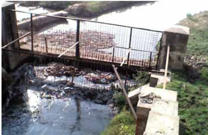
Existing Coarse Screen at Morigate Pumping Station
