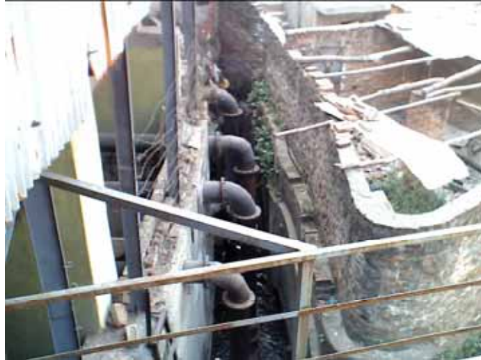
Morigate Pumping Station
