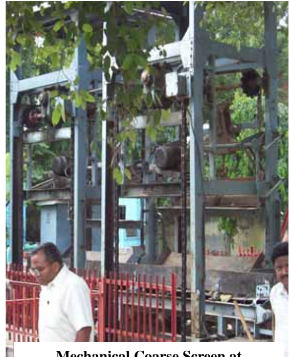
Mechanical Coarse Screen at Gaughat SPS – Non Functional
