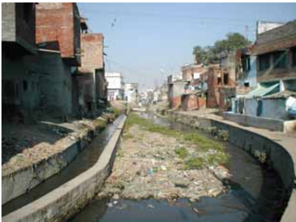
Photo 6.7 Garbage with Sediment Forming Sandbar in Nala (Wazirganj Nala, Lucknow)
