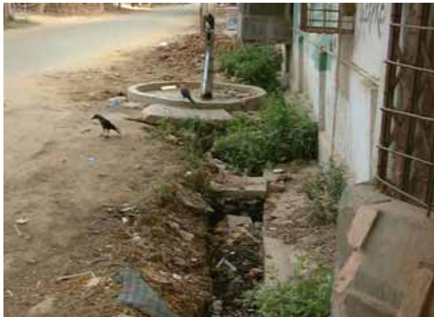
Photo 2.3 Condition of Small Street Gutter
