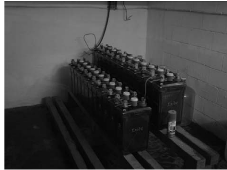
Battery of communication system
