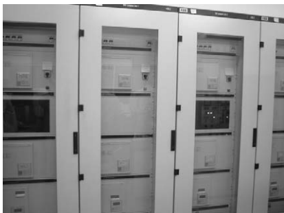
Control Board of Transmission/Line
