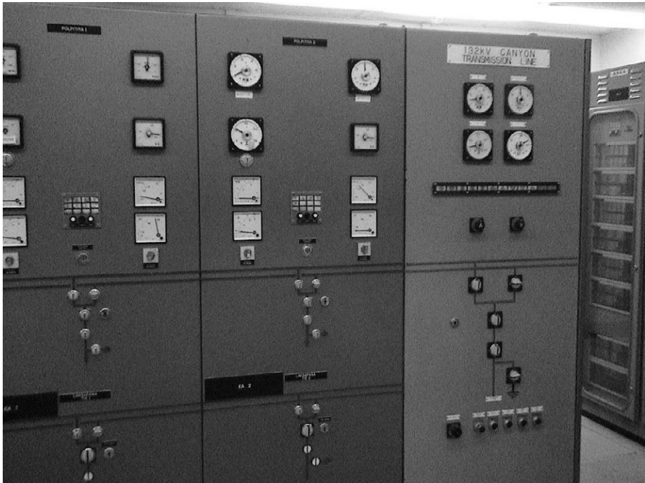
Control boards of transmission line
