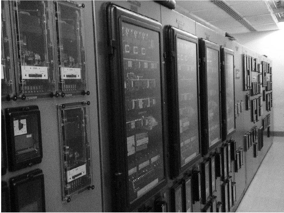
Protection relay boards
