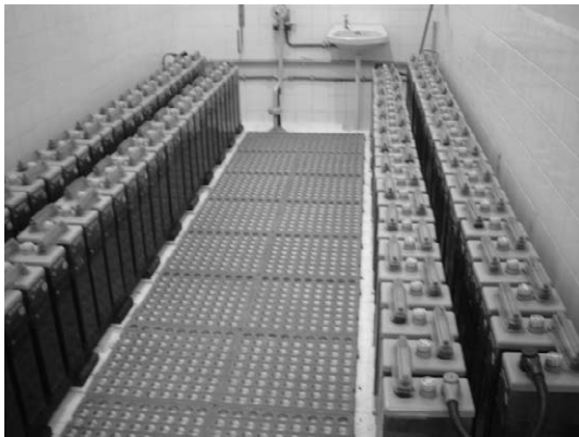
Battery of control system
