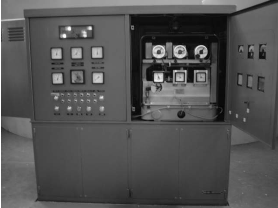
Governor & Actuators cubicle
