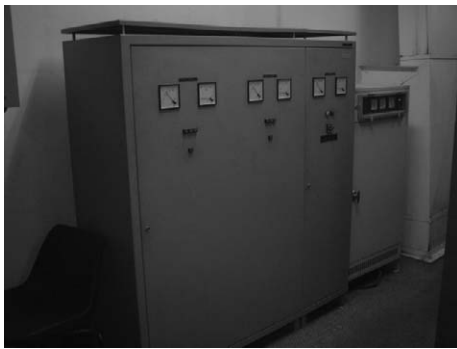
Battery Charger Cubicles of Communication
