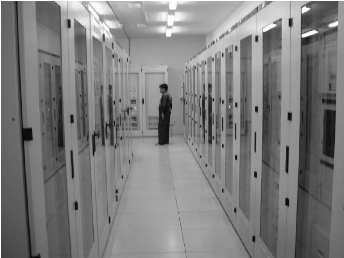
Control Boards of Generator / Transformer (left site) and Transmission Line (right side)
