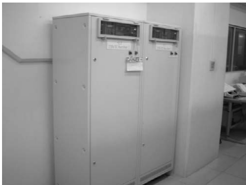
Battery Charger of Control
