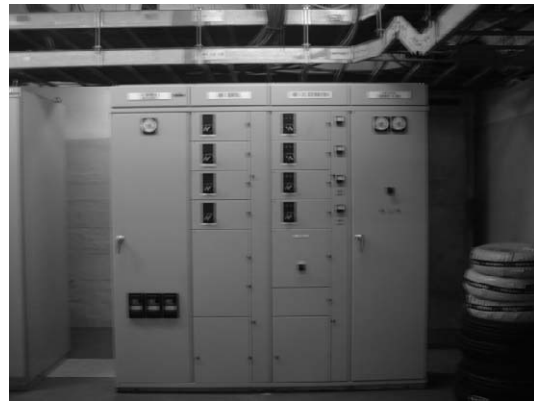
Motor control center (MCC)
