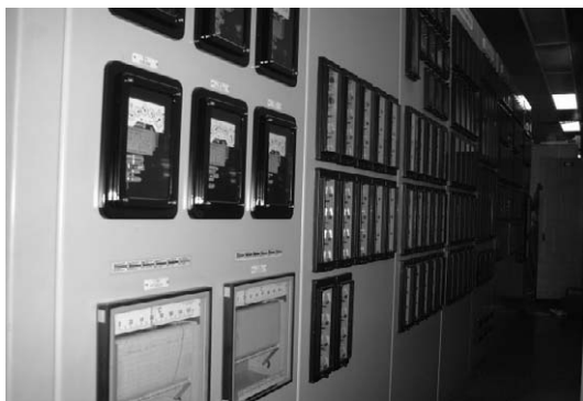
Protection relay boards
