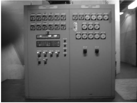
Turbine control & actuator cubicles
