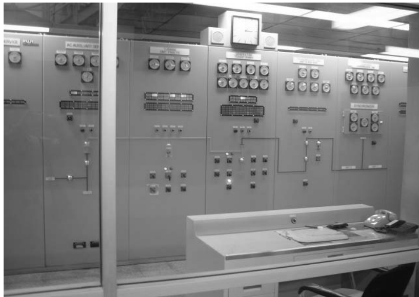
Unit 1 main & station service control board
