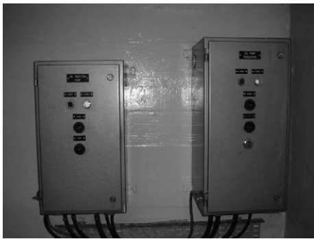
Compressor control panel
