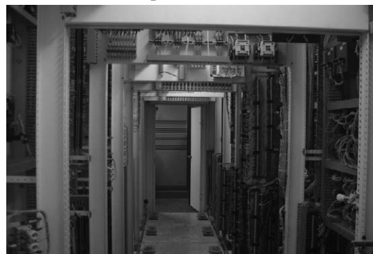
Inside of both control & protection boards
