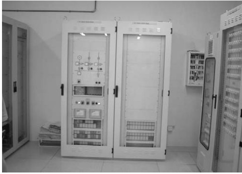
Station Service Boards
