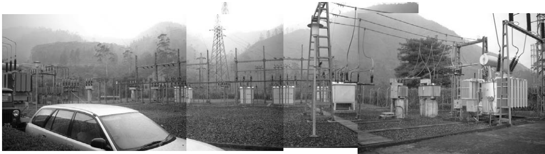
3.3 kV Switchgear & Distribution Line
