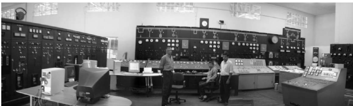
Computer control with CRT shown on left side and Remote control desk for New-Laxapana PS (right side) (Old control boards <black color>)
