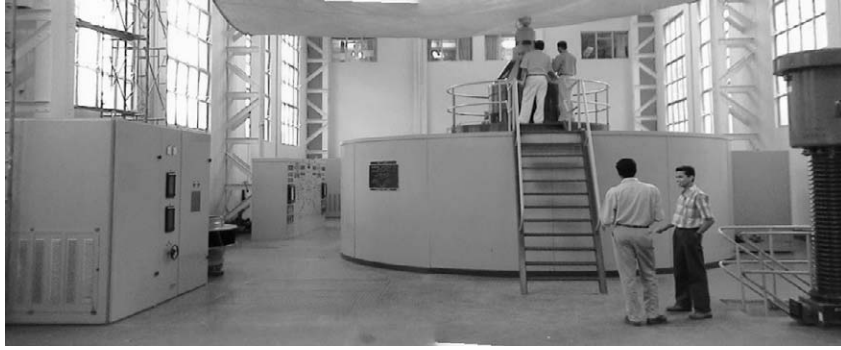
Generator and Excitation Cubicles (left side)
