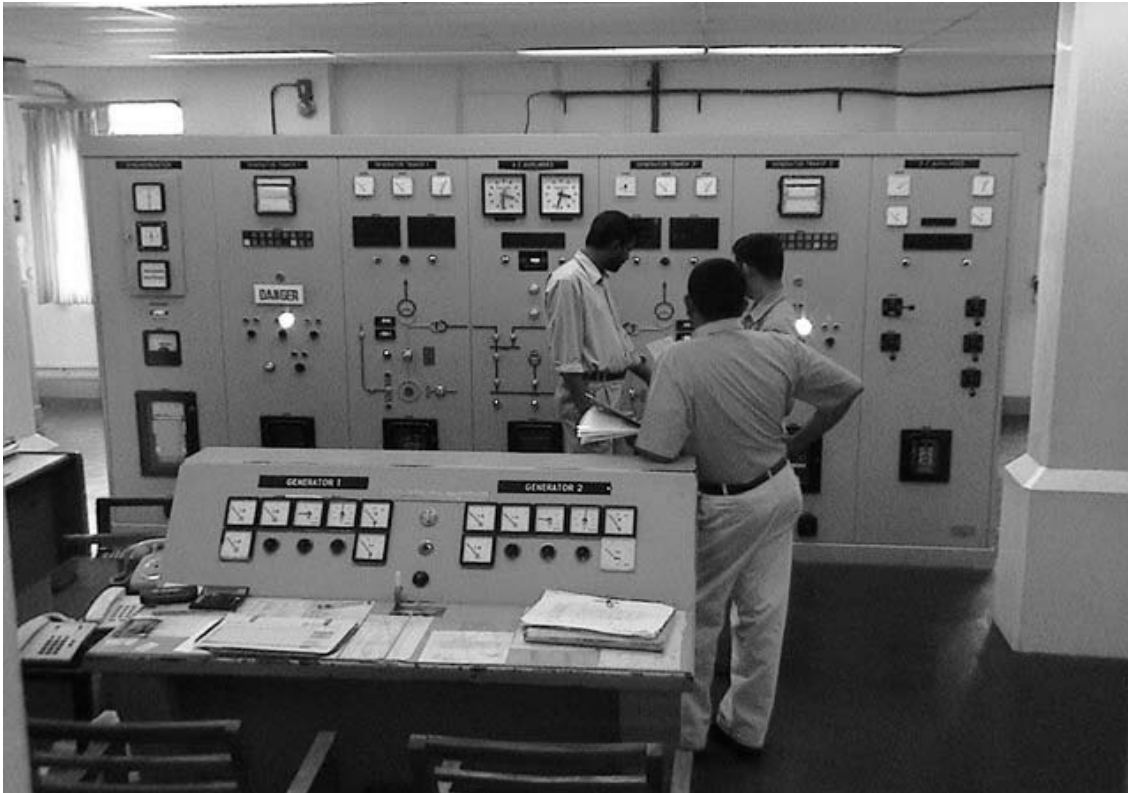
Main Control Board and Control Desk
