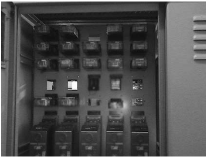
Auxiliary Relay in Board
