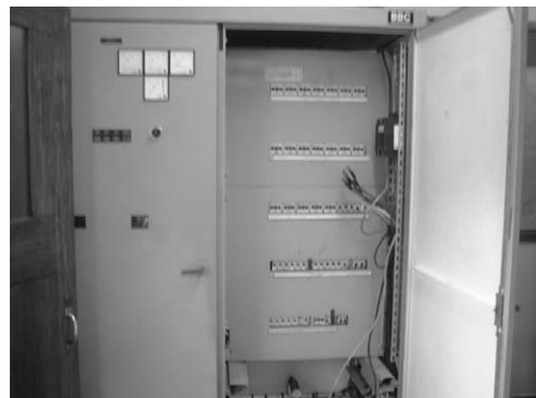
DC Distribution Cubicle
