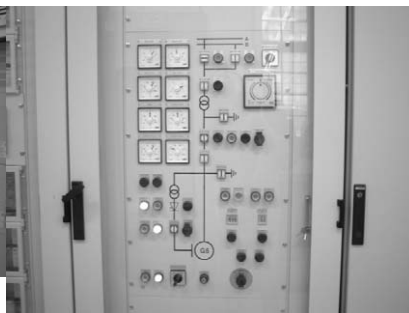
Local control board
