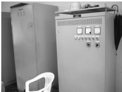
Battery Charger Cubicle
