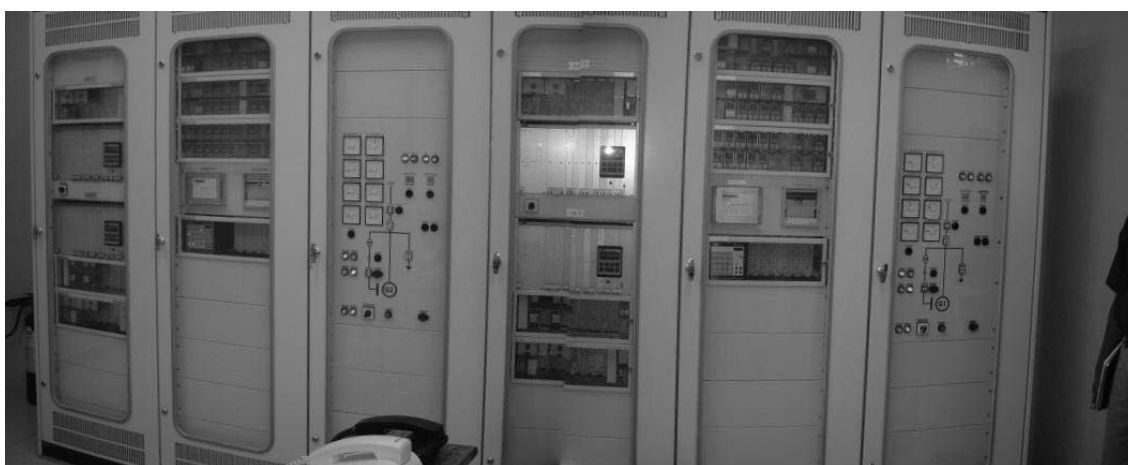
New Control Boards of Units 1 & 2 renewed by 2003
