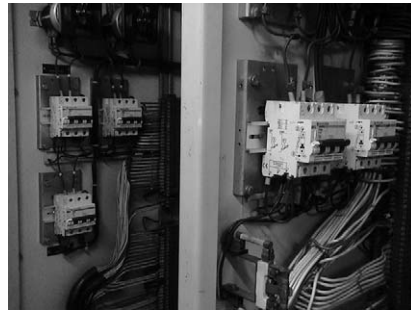
Renewed No Fuse Switch
