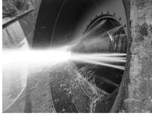
Picture 6.4 Leakage from needle valve
