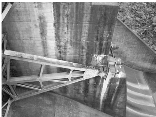
Picture 6.25 Trunnion requires access facility
