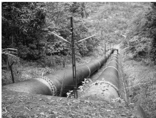
Picture 6.21 Panorama view of penstock
