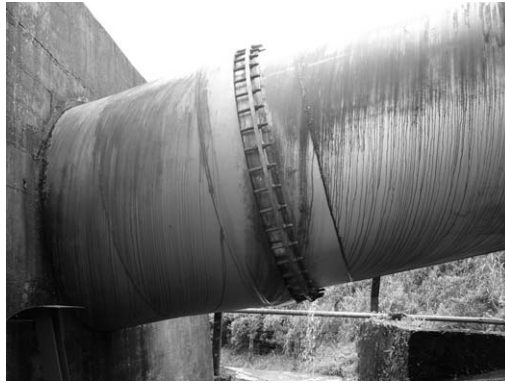
Picture 6.12 Leakage from expansion joint
