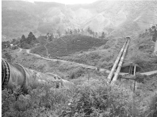
Picture 6.1 Panorama view of penstock
