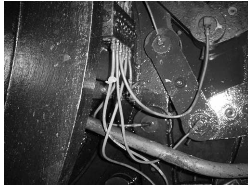
Picture 7.8 Crack in Guide Ring for Wicket Gate Operating Mechanism of Polpitiya Turbine
