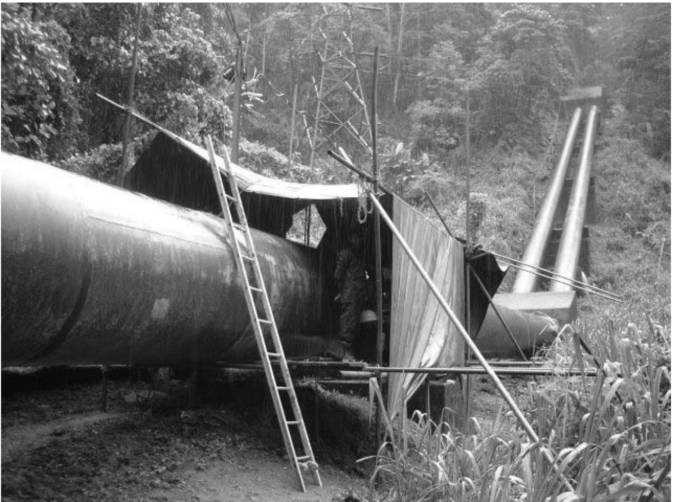
Efficiency test in New Laxapana Hydropower station
