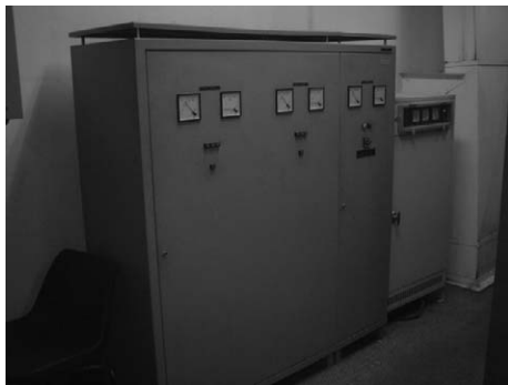
Battery Charger Cubicles of Communication
