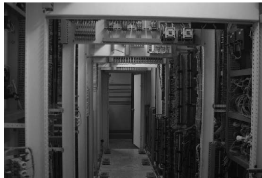
Inside of both control & protection boards
