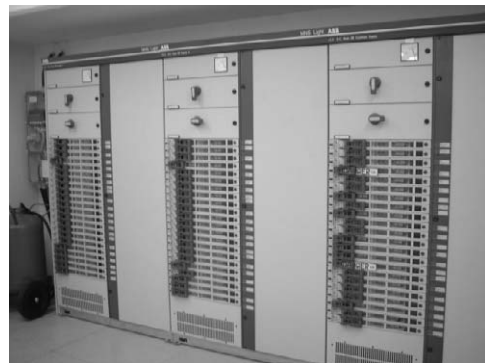
DC Distribution Boards
