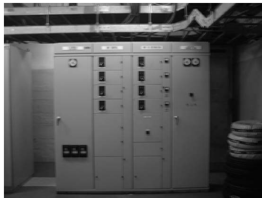
Motor control center (MCC)
