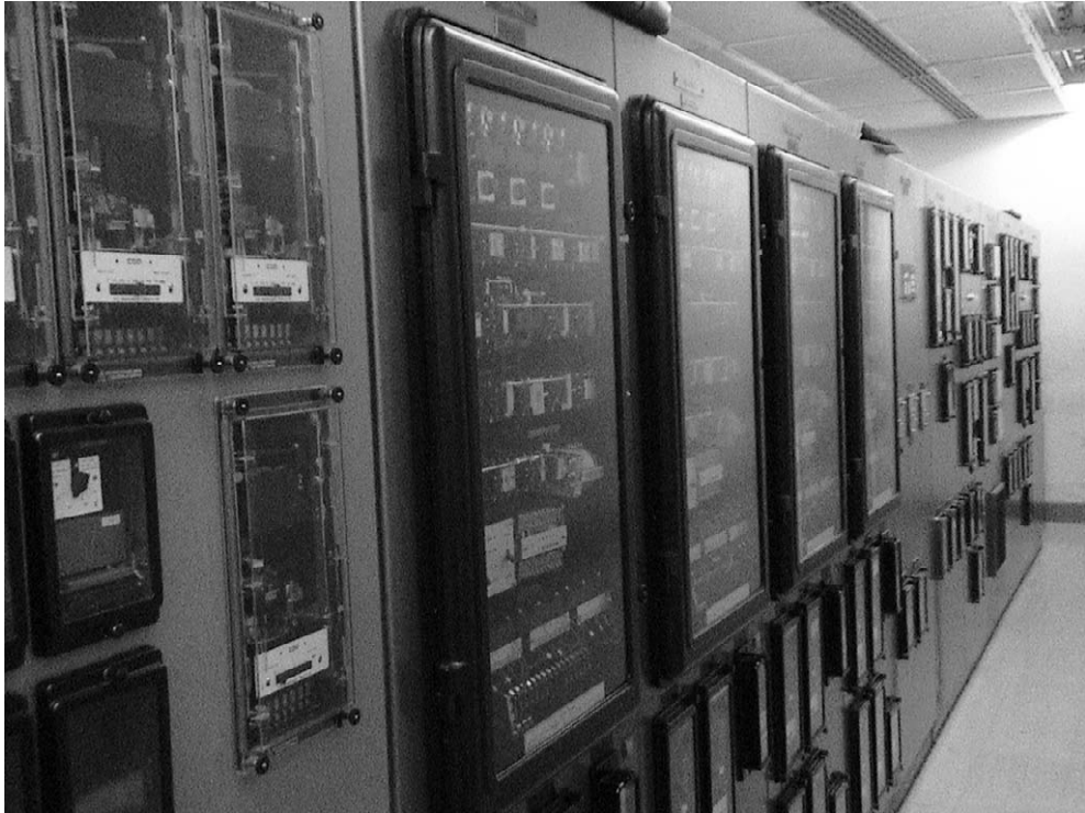
Protection relay boards
