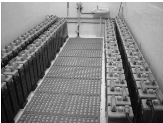
Battery of control system
