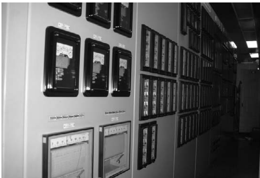
Protection relay boards
