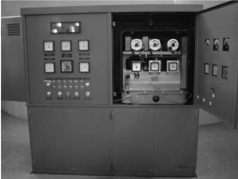
Governor & Actuators cubicle
