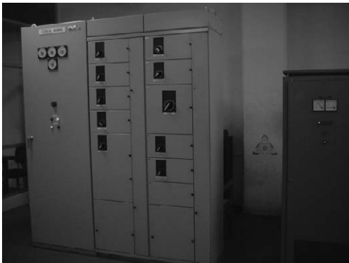
DC distribution board
