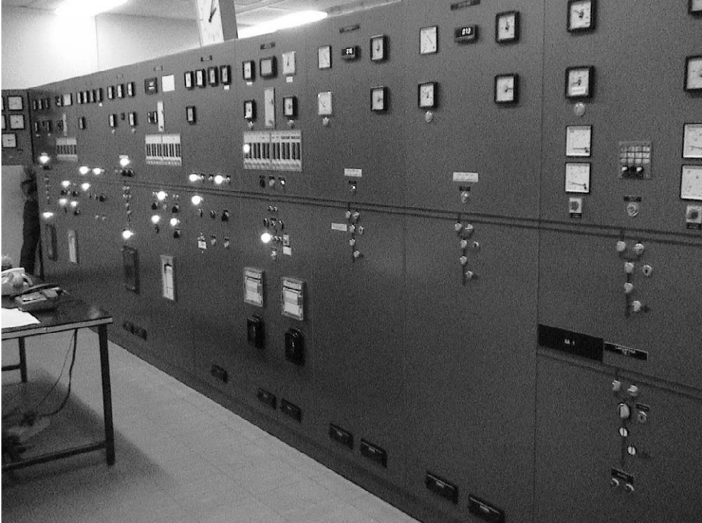
Control boards of turbine- generator and transmission line
