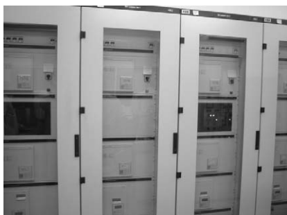
Control Board of Transmission/Line
