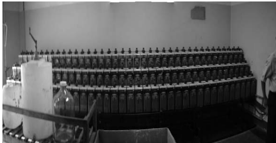
Battery (110VDC) of control system
