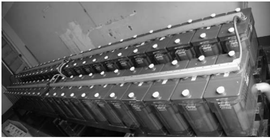
Battery (48VDC) of communication system
