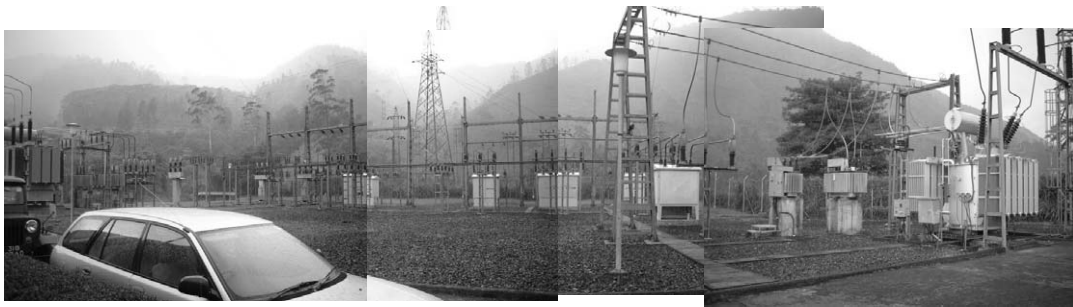
3.3 kV Switchgear & Distribution Line
