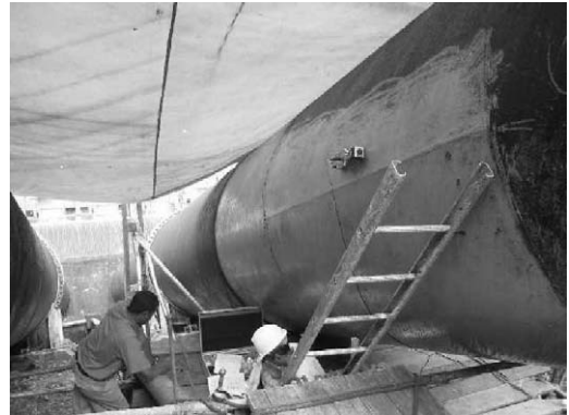
Picture 1 Sensor installation state
