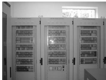
Aux. relay boards
