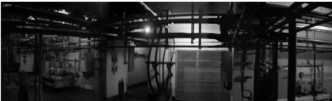
Control cables in cable treating room Control cable arrangement under floor of turbine-generator
