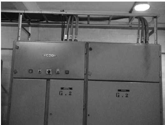
Excitation Equipment Board
