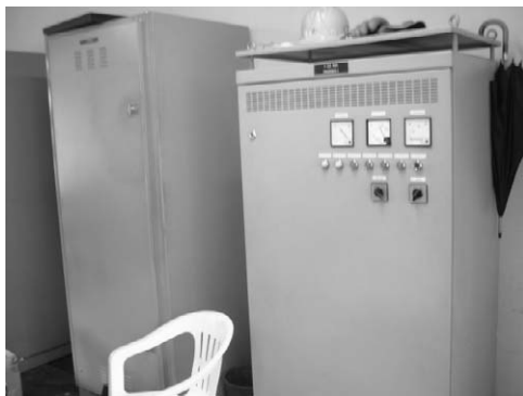
Battery Charger Cubicle
