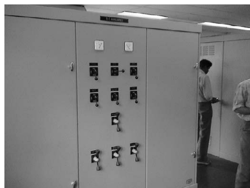
DC Auxiliary Board
