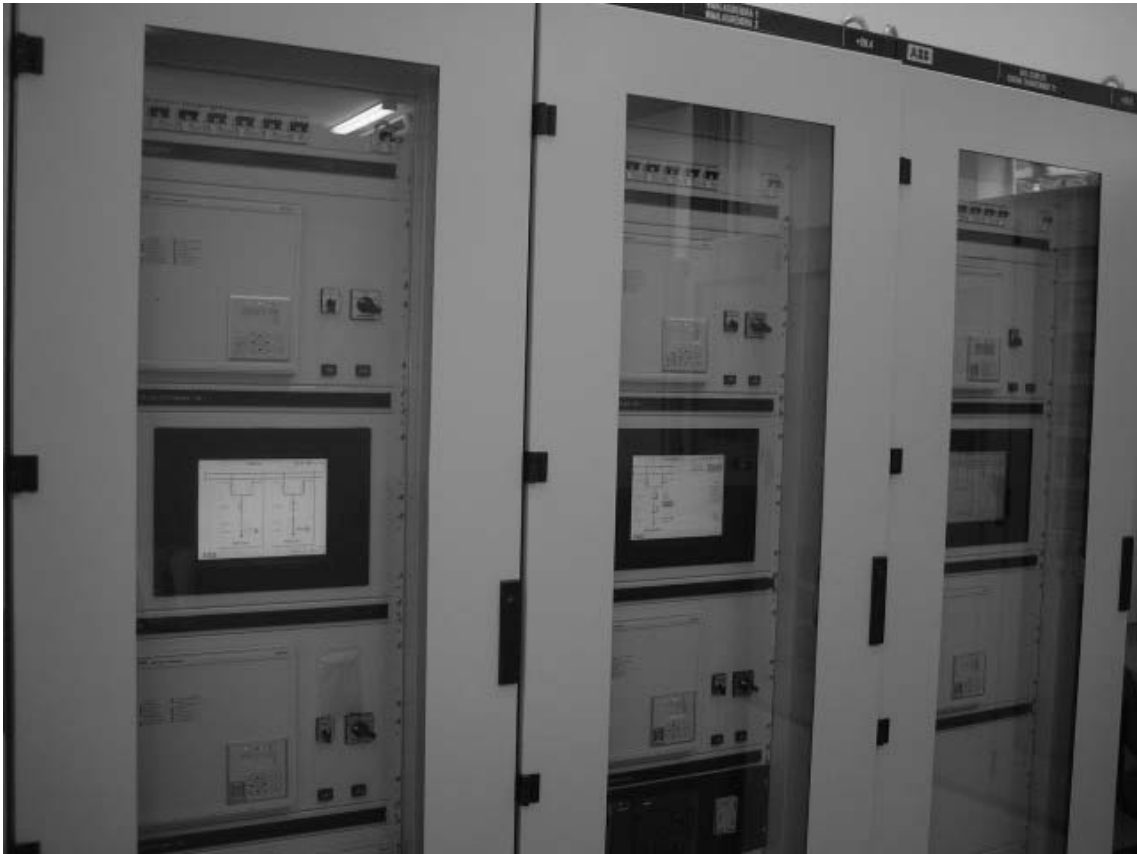
Control & protection relay boards of transmission line
