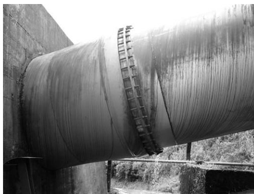
Picture 6.12 Leakage from the expansion joint
