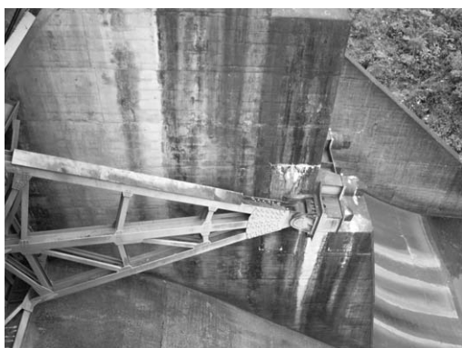
Picture 6.25 Trunnion requires access facility
