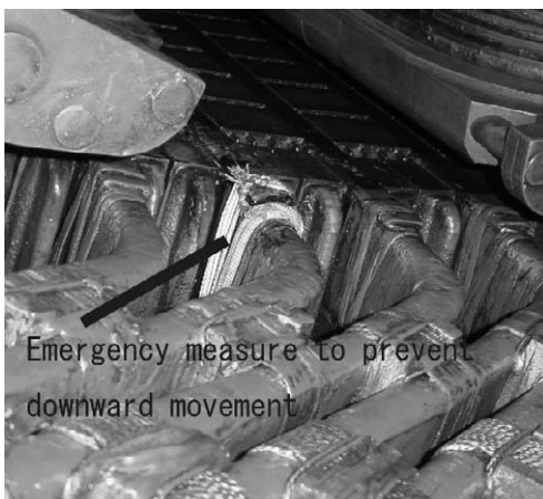
Picture 7.1 Present status of the stator in Unit 1
