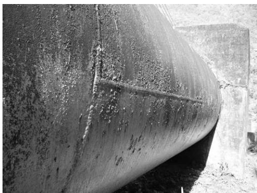
Picture 6.23 Outside surface of welded joint
