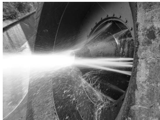
Picture 6.4 Leakage from needle valve
