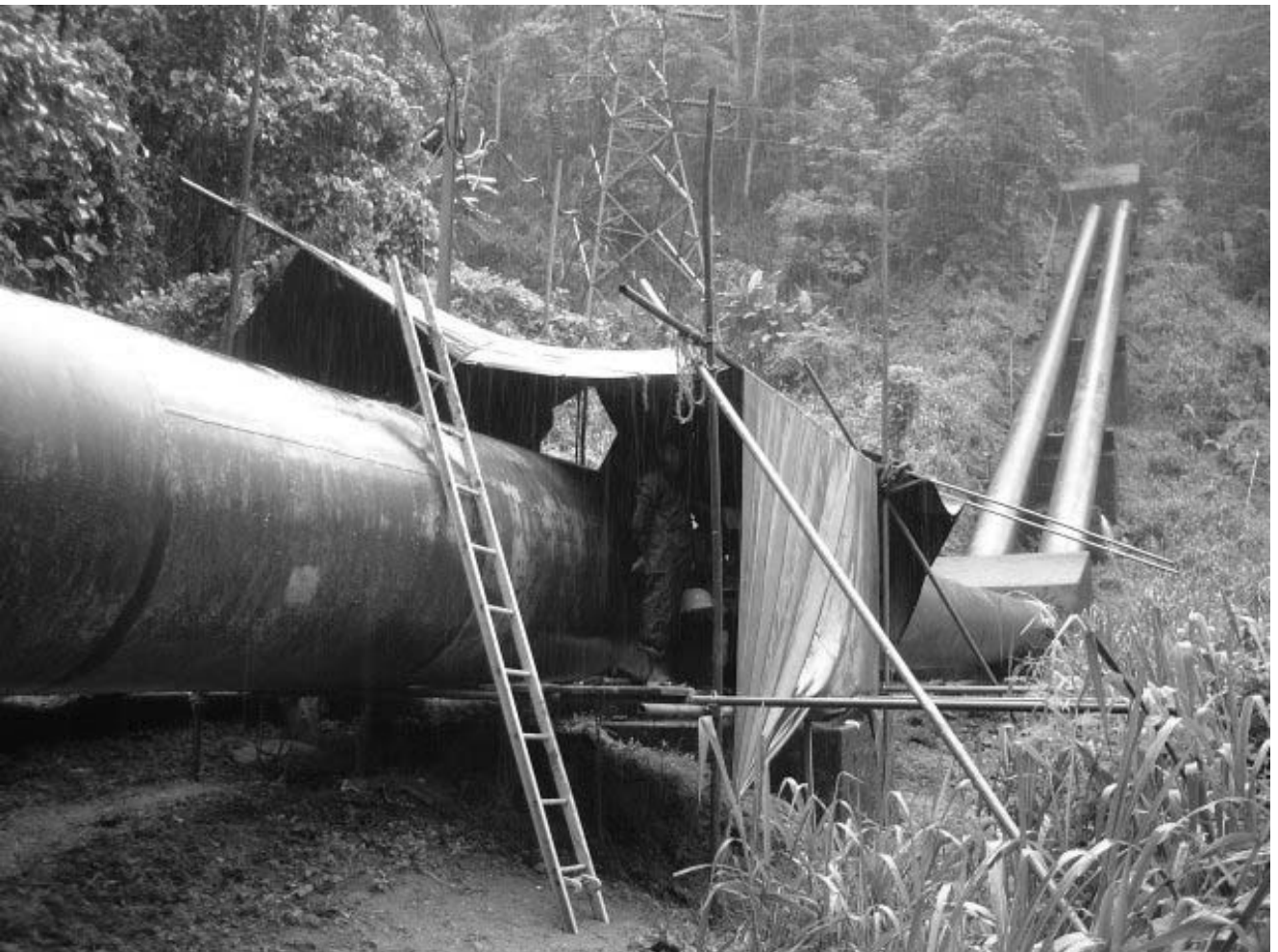
Efficiency test in New Laxapana Hydropower station
