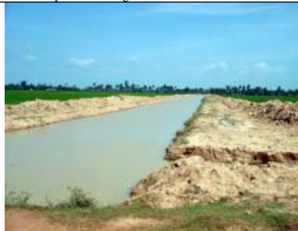
Photo-5: The Lumbach main canal of Ou Krang Ambel irrigation system. The main canal was connected with the existing main canal in the downstream to command paddy field in Angk Snuol District of Kandal. The connecting canal was constructed by Western Phnom Penh Integrated Area Project in 2003.
