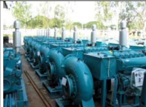
Photo-9: Diesel engine pumps of MOWRAM (Dept. of Irrigated Agriculture). MOWRAM has its own workshop to assemble the pump set for irrigation system. Pump irrigation is widely used in gravity irrigation scheme for "intervention" during emergency dry period.
