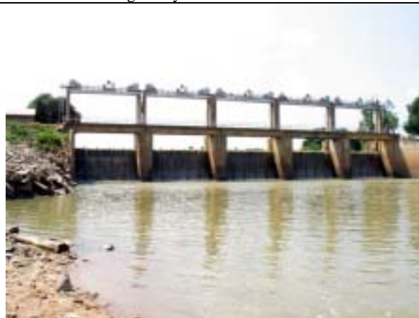
Photo-6: Nov.19,2003. Roleang Chrey Regulator. Over flow depth was 0.12 m (WL=7.12 m). Generator, motor, cable for the gate, and others are considered to be upgraded or replaced.
