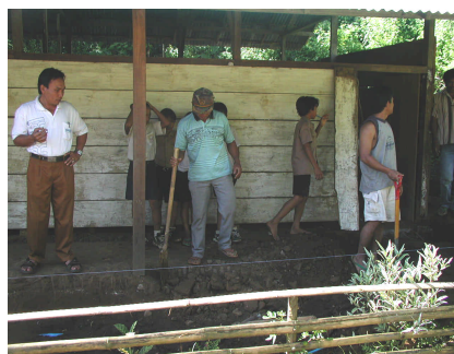
<Left> Community residents work for classroom rehabilitation (SLTP Swakarya Powaltan, Kab.Minahasa, North Sulawesi)
