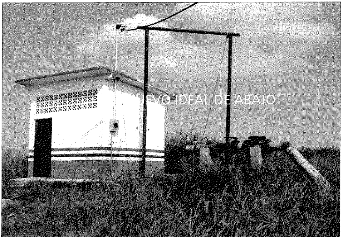
PUMPING STATION IN THE WELL 28 SUBMODULE
