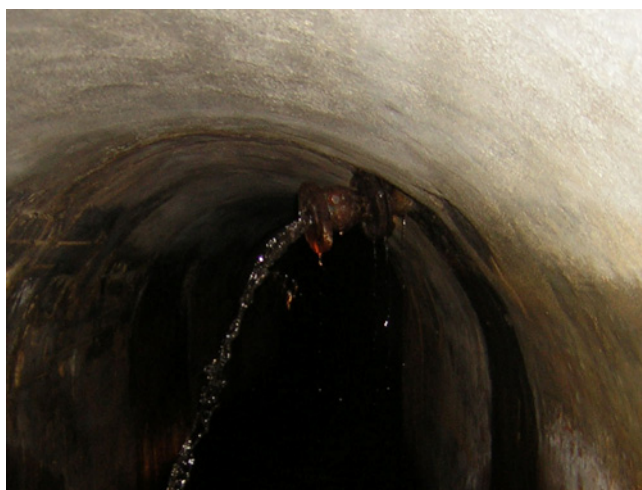
Figure2.1 Water Flooding into Old Tunnel at TD977.5
