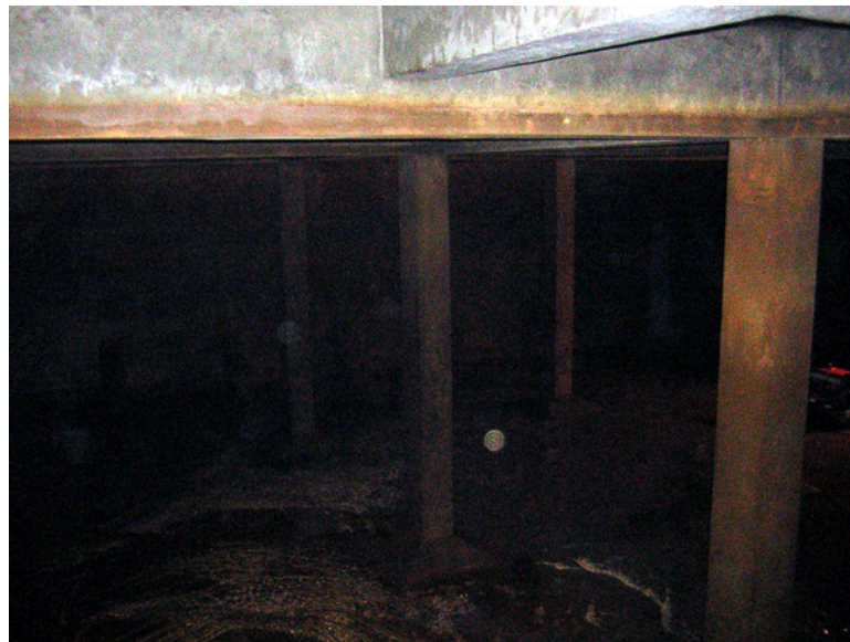
Figure1.6 Old Wali Reservoir (a photo taken from old tunnel exit to the reservoir)
