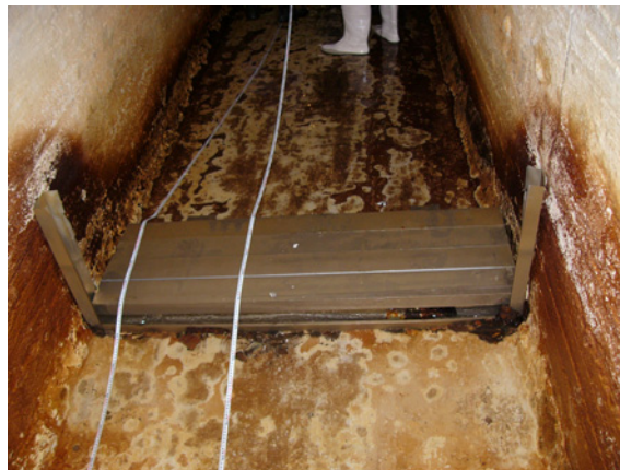
Figure 1.5 Simple Weir inside Old Tunnel (about TD290)
