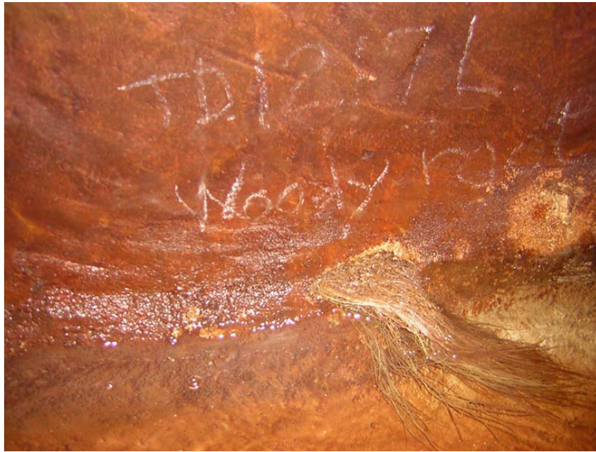
Figure1.17 Penetrated Roots into Old Tunnel at TD 1217
