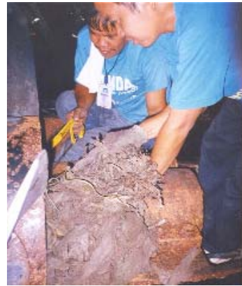
Plastics tangled around Pump Shaft
