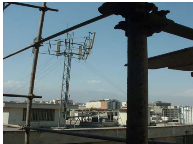
Figure 11.1.5 GSM Antenna Fixture in Guyed Tower
