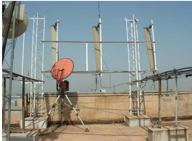
Figure 11.1.4 GSM Antenna Fixture in Roof Wall
