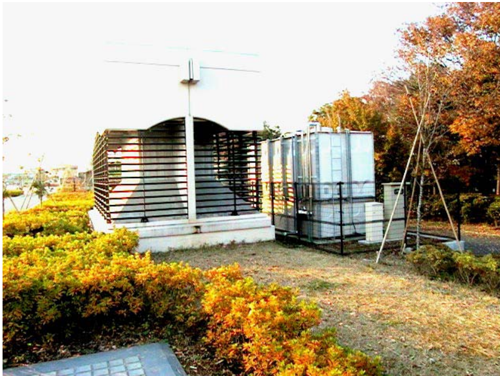
Figure 11.7.4 Example of Emergency Water Facility
