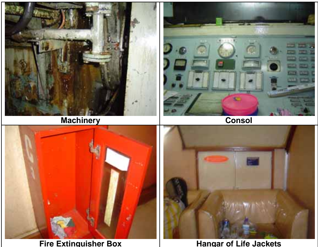
Photo 5.1.1 Examples of Non-conformities which are Solvable Only Crew's Effort
