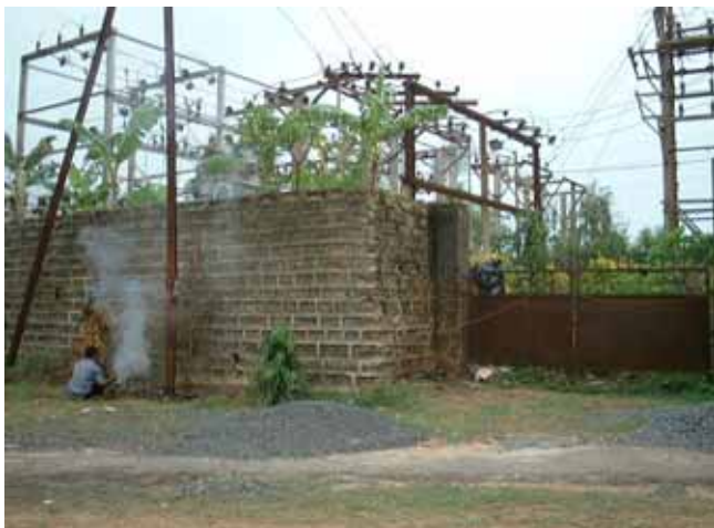
ELECTRIC CORPORATION'S SUBSTATION
