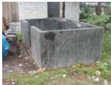
Ash storage container
