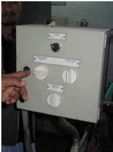
Switch box for furnace operation
