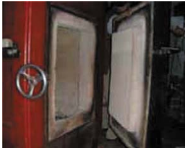
Waste charging door
