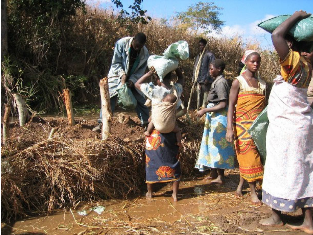
An example of constructing a diversion weir: No machinery is employed in constructing smallholder irrigation facilities. Villagers, women as well as men, participate in the construction and they can finish within one day in most cases.
