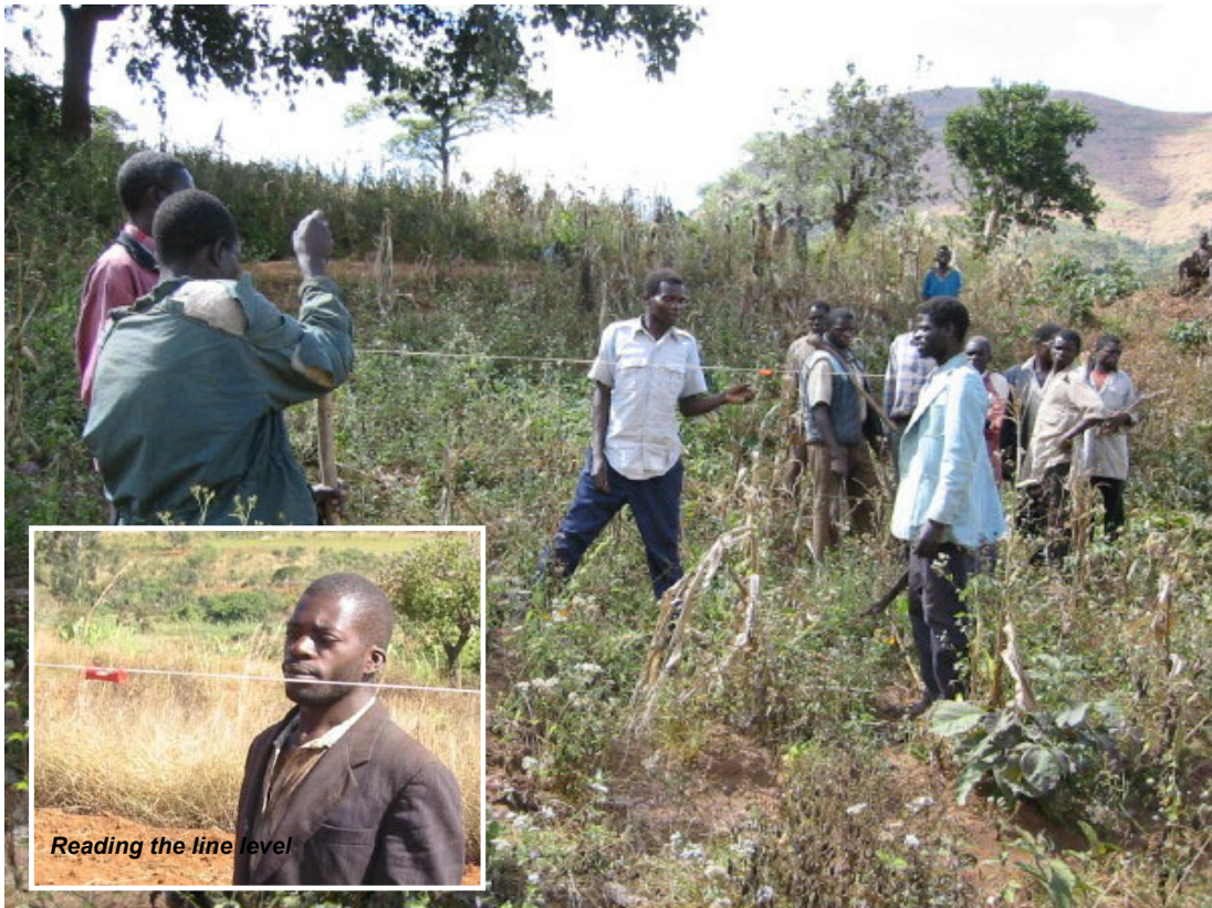
Canal alignment by using a simple tool that is, line level: Sprit line level is used in aligning canal according to the contour of the topography. Villagers can get used to handling of the line level in half an hour given on-the-job-training.
