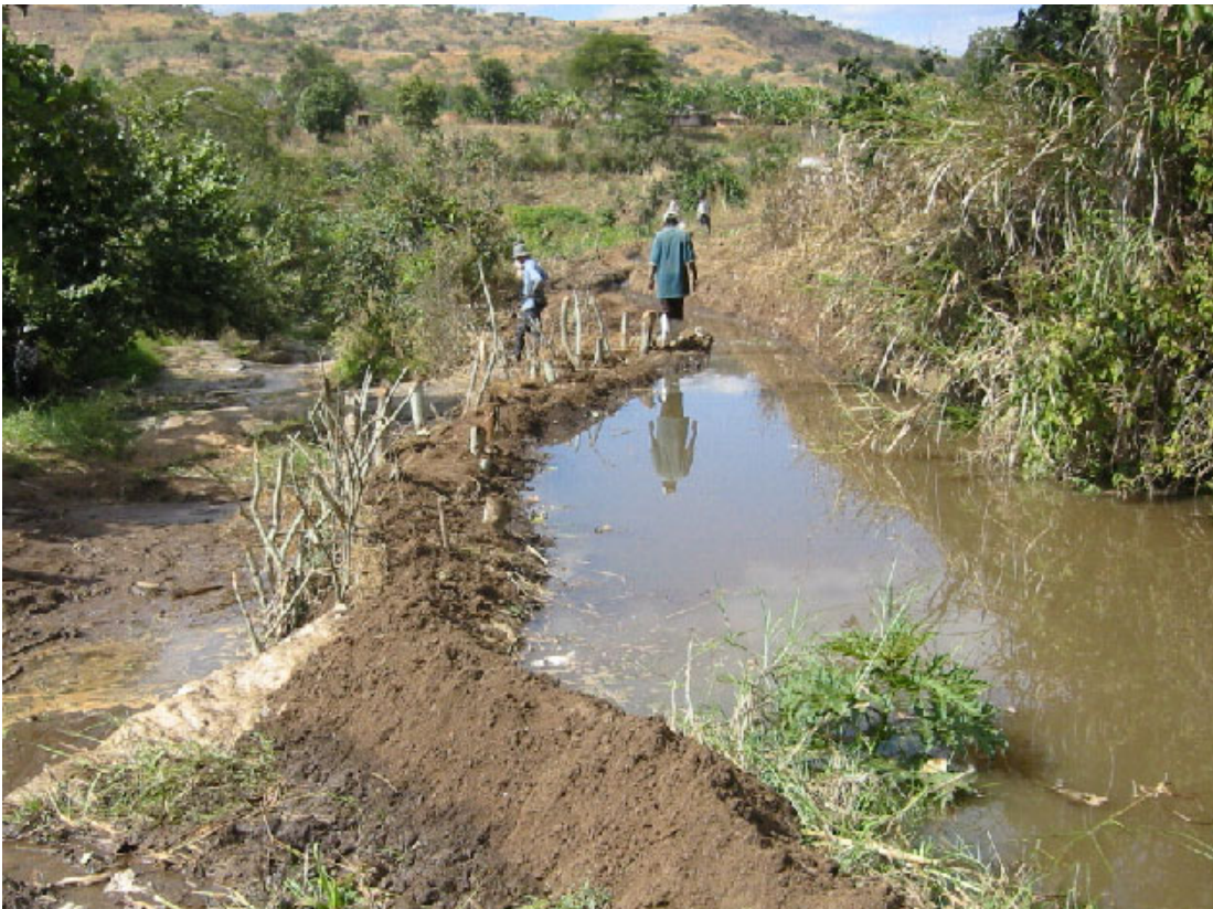
Completion of the diversion weir constructed by the villagers shown in above photo: This weir has double fences, made out of wooden poles and woven grasses, in which clay soil is compacted so that leakage can be minimized while raising the water level.
