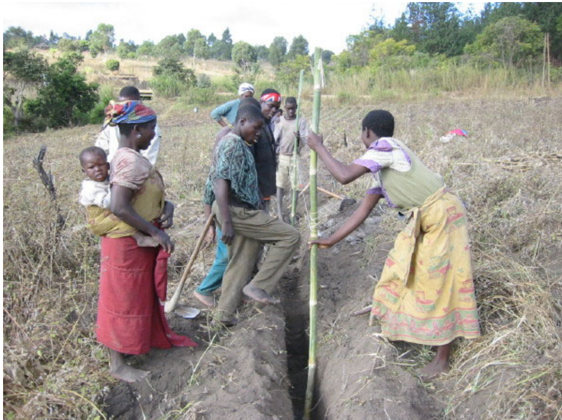
Gradient checking by using the line level: After excavating the canal aligned with the line level, they check the longitudinal gradient of the canal by using the same line level in order for the water to be assured to run smoothly by gravity.
