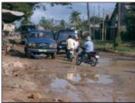
Figure 15-35: Damaged road during rainy season
